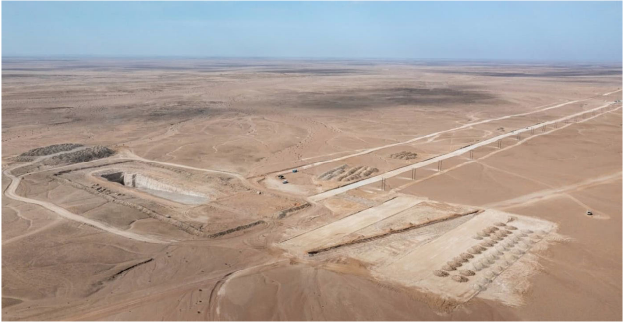
Figure 2: Significant progress continues on bulk earthworks at Etango, a key enabler of future construction and development activities. The primary crusher has been fully excavated and its dimensions confirmed, while work advances on the permanent road and conveyor belt line to the secondary and tertiary crushing areas.
