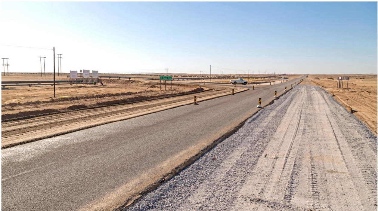
Figure 6: Widening of C28 intersection entrance area to improve safety as vehicles enter site access road.
