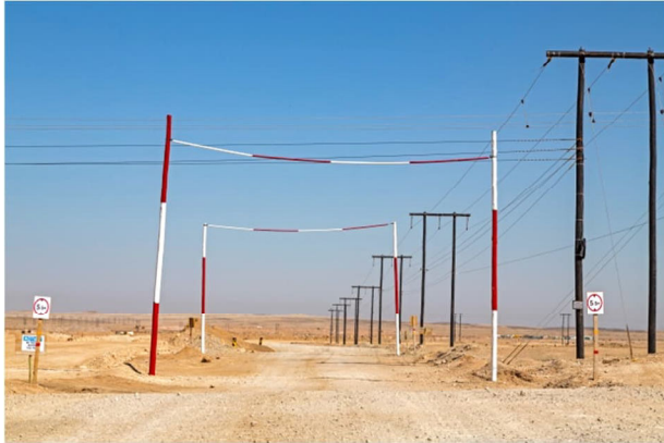
Figure 4: Power grids on site are now live with safety precautions to prevent vehicles crossing under installed lines
