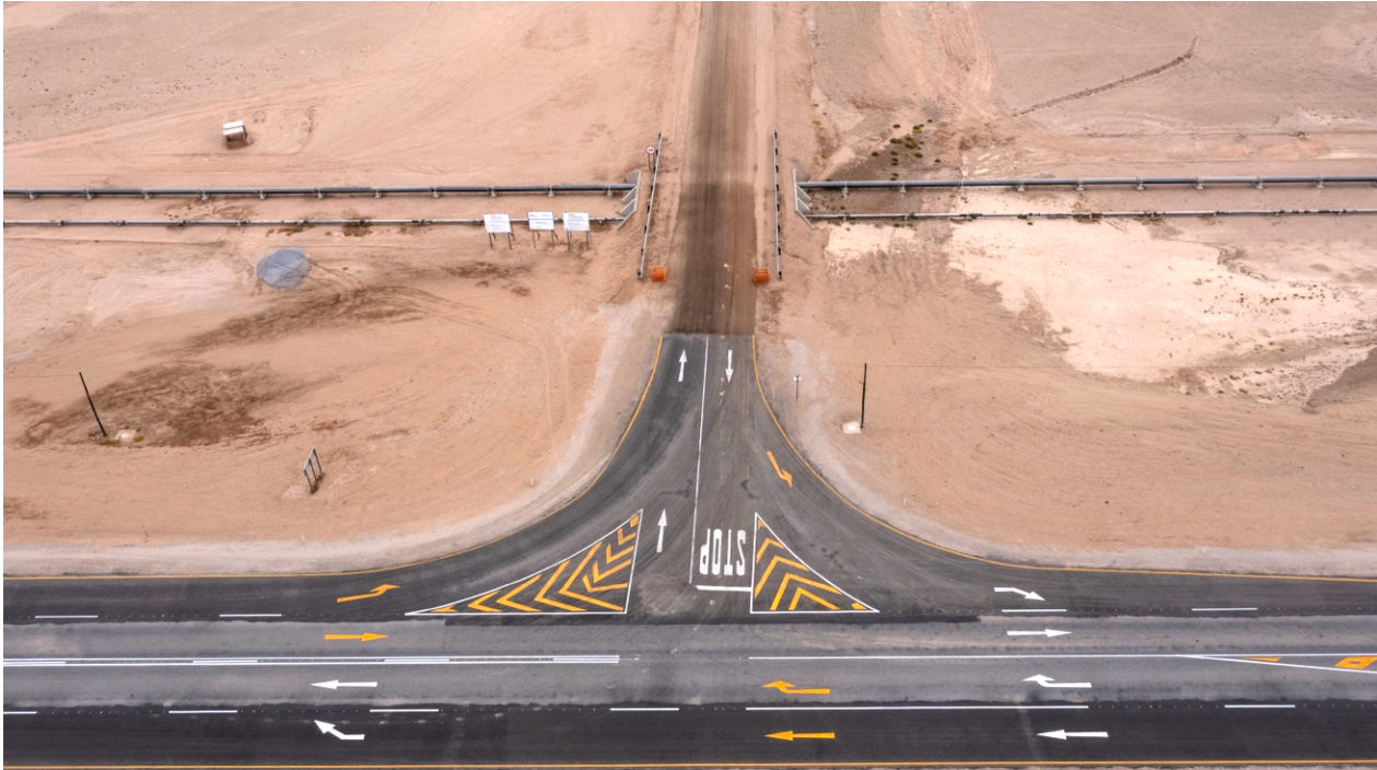
Figure 2: Widening of the C28 intersection entrance area is complete, improving safety as vehicles enter site access road.
