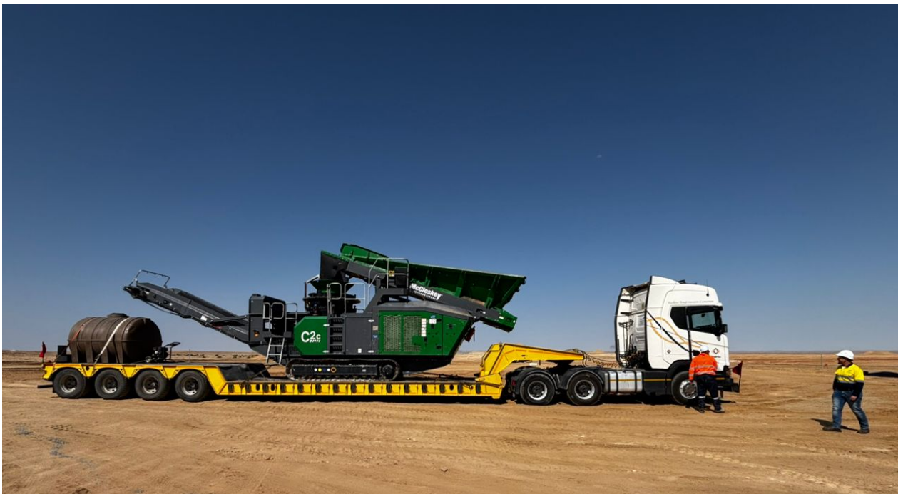
Figure 3: The first crusher has arrived onsite at Etango for the crushing of aggregate for the heap leach drainage layer.
